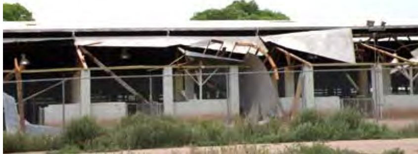
Wind damage, County Fairgrounds, 2012
