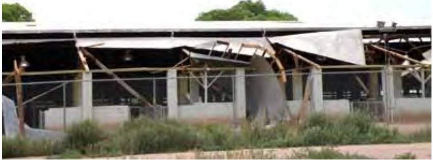
Wind damage, County Fairgrounds, 2012
